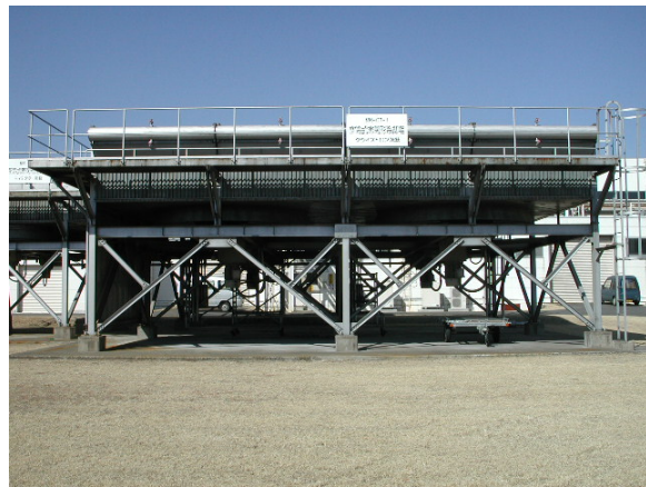
Air cooled heat-exchanger
