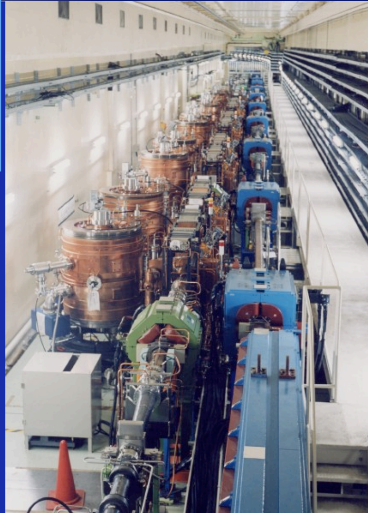
ARES cavities in the LER RF section Fuji D7
