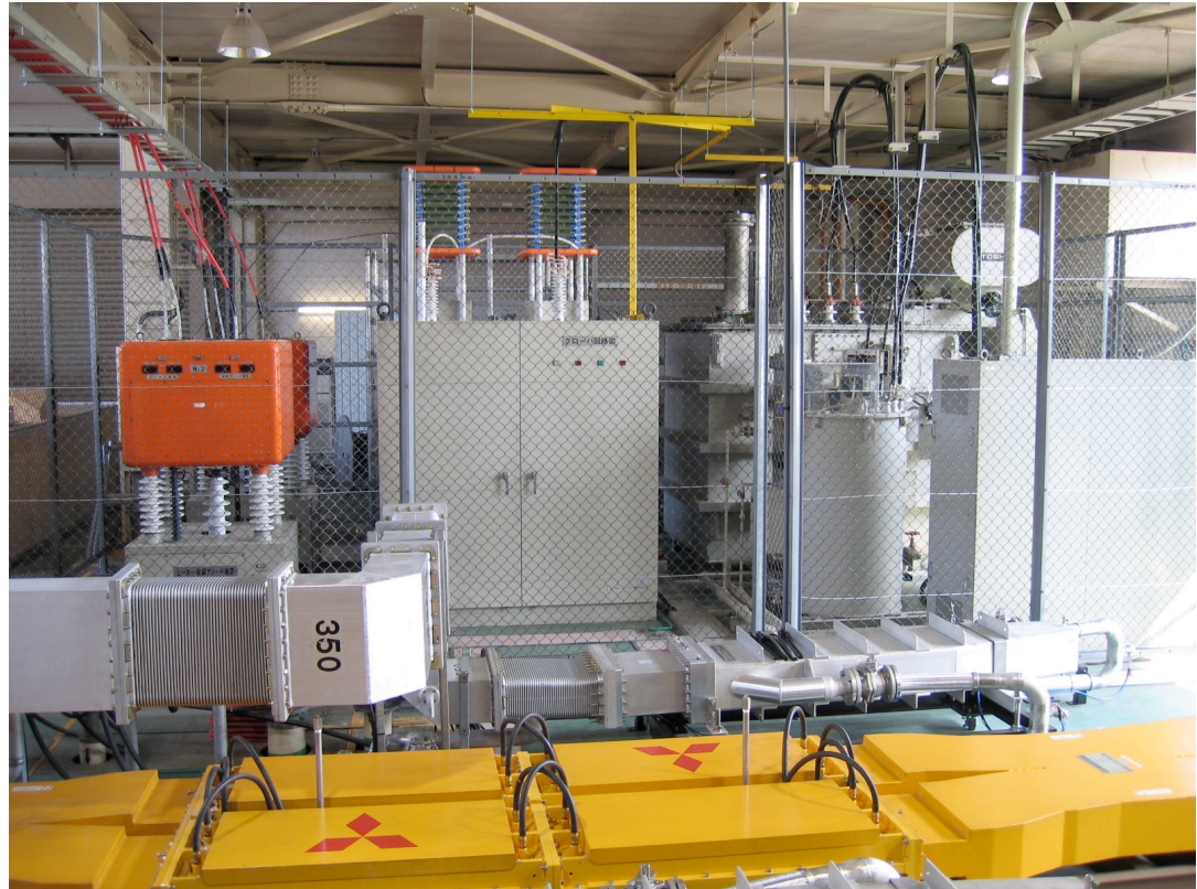
Power supply for the klystrons Circulator and dummy load
