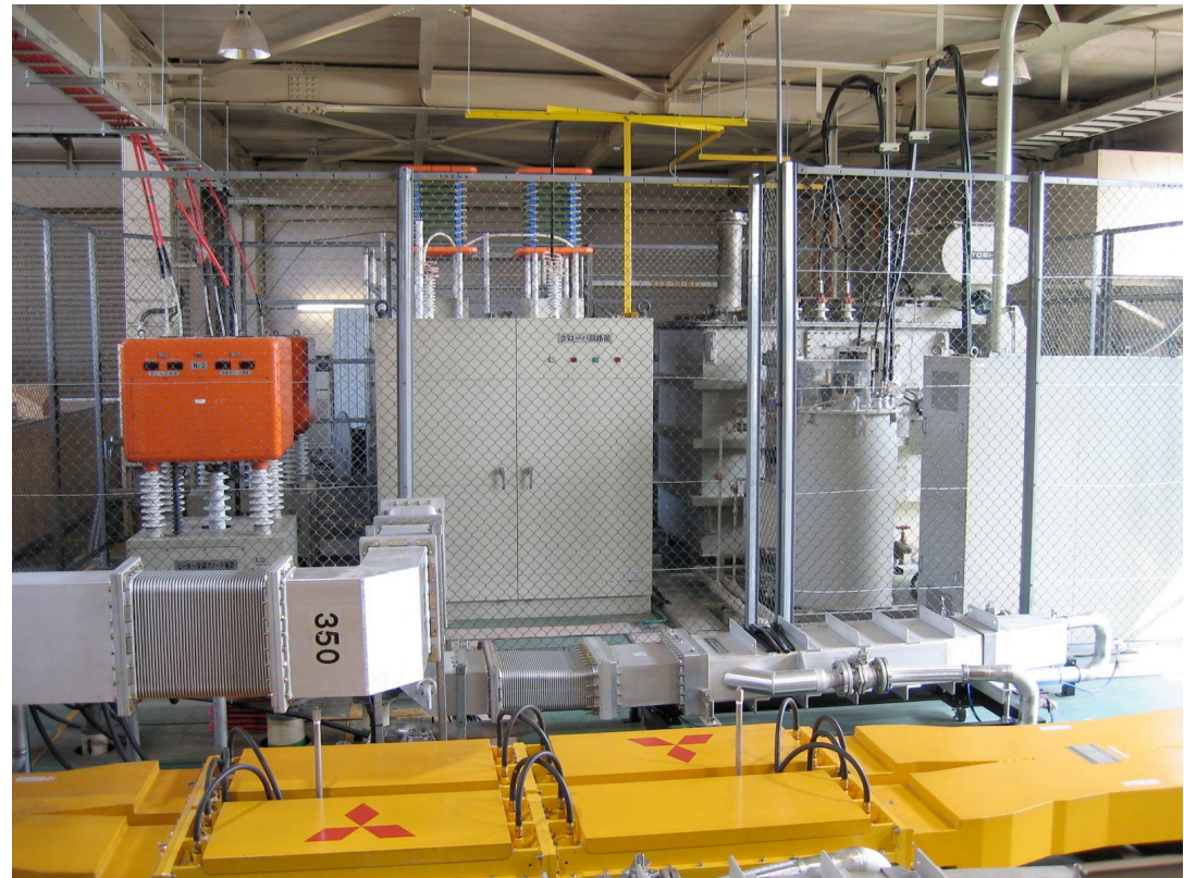
Power supply for the klystrons
