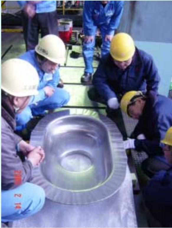
Forming of 4 Half-Cells for Crab # LER and # HER Finished on Feb. 14, 2005 at Mitsubishi Heavy Industries, LTD. Kobe
