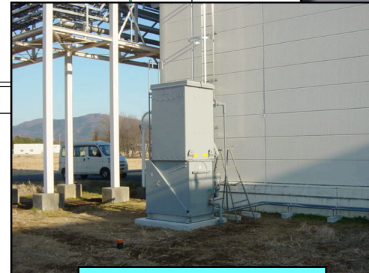
Cooling Tower 68 kW
