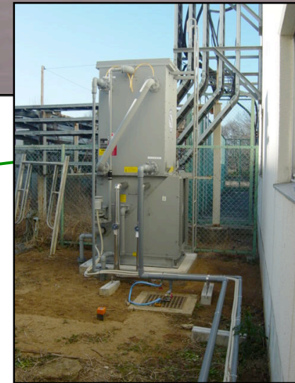
Cooling Tower 68 kW
