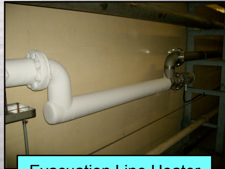
Evacuation Line Heater
