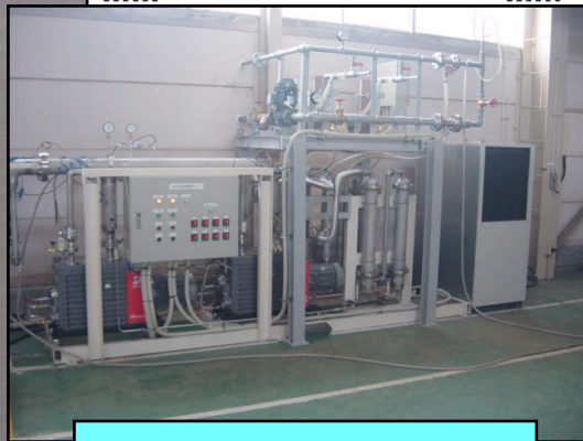
Evacuation & Chiller Units
