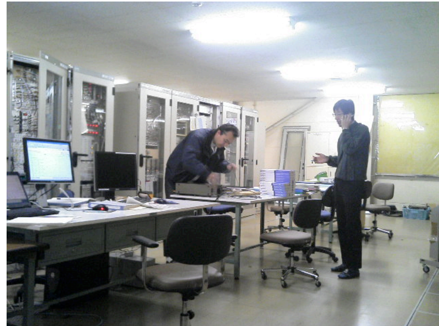
Control system at D11 station
